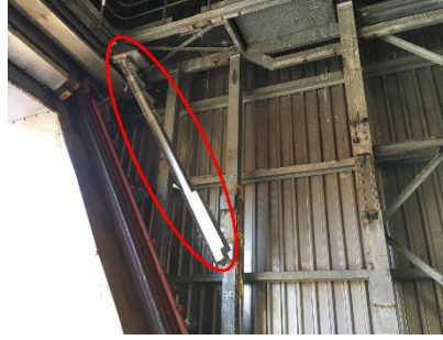
Fig. 2: Picture of the scanning bar (surrounded in red) installed at the receiver aperture before the installation of the receiver
