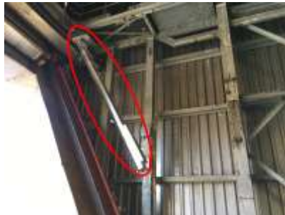
Flux measurement system installed (moving bar surrounded in red)
